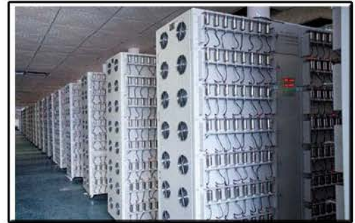
Cell Batching and Monitoring Stations
